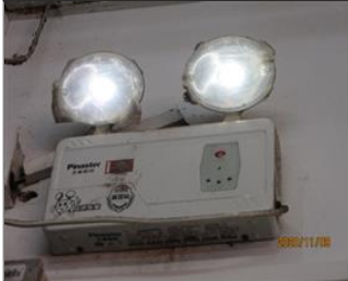
External photo(s) of the production unit(s) NO-21 Emergency light testing.JPG
