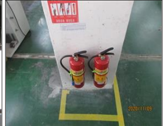
External photo(s) of the production unit(s) NO-23 Fire extinguishers.JPG
