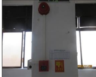
External photo(s) of the production unit(s) NO-22 Fire alarm.JPG
