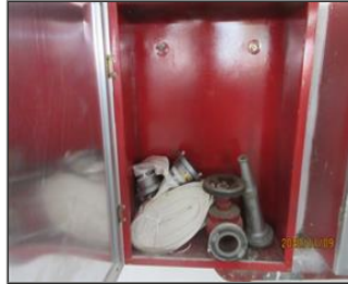
External photo(s) of the production unit(s) NO-25 Fire hydrant.JPG
