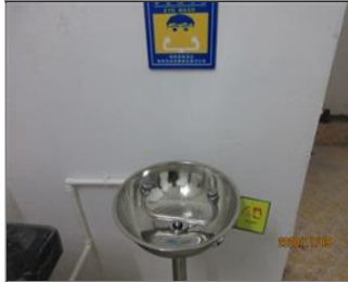
External photo(s) of the production unit(s) NO-16 Eye washing facility.JPG
