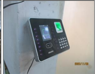
External photo(s) of the production unit(s) NO-9 Attendance recording system.JPG
