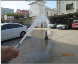
External photo(s) of the production unit(s) NO-24 Fire hydrant testing.JPG
