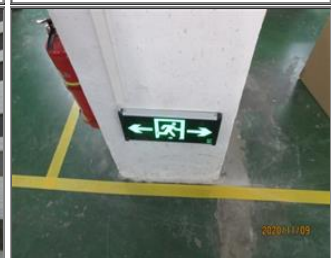
External photo(s) of the production unit(s) NO-20 Evacuation sign.JPG
